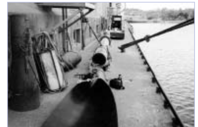
Agricore staff manually rolled the TIVAR® 88-2 antistatic liner and clamped it with a steel collar.
