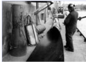
Ropes and the steel collar guide the TIVAR® 88-2 liner into the pipe.
