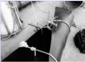
The steel collar devised to help roll the liner at it's pulled into the pipe.
