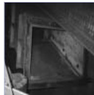
Original rectangular shape transfer chute.
